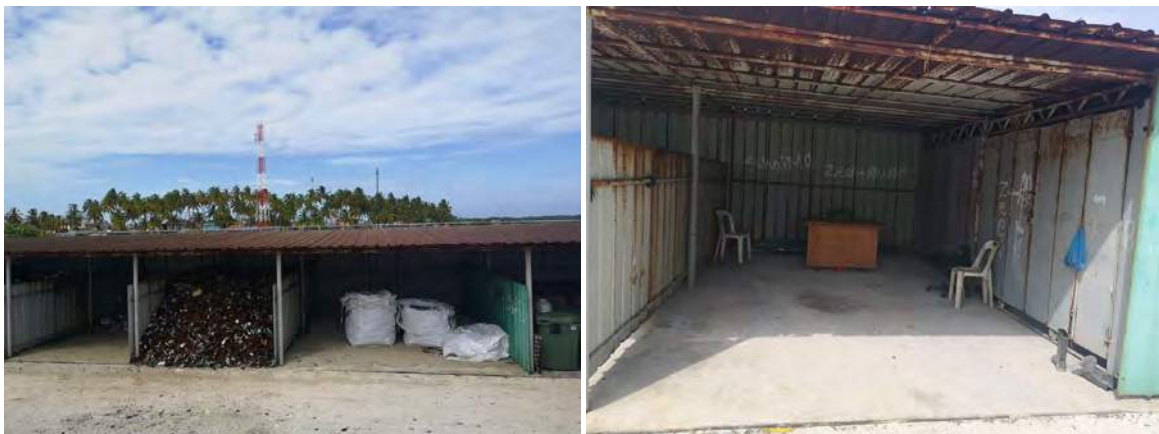
Figure 11 Waste sorting area severely rusted
