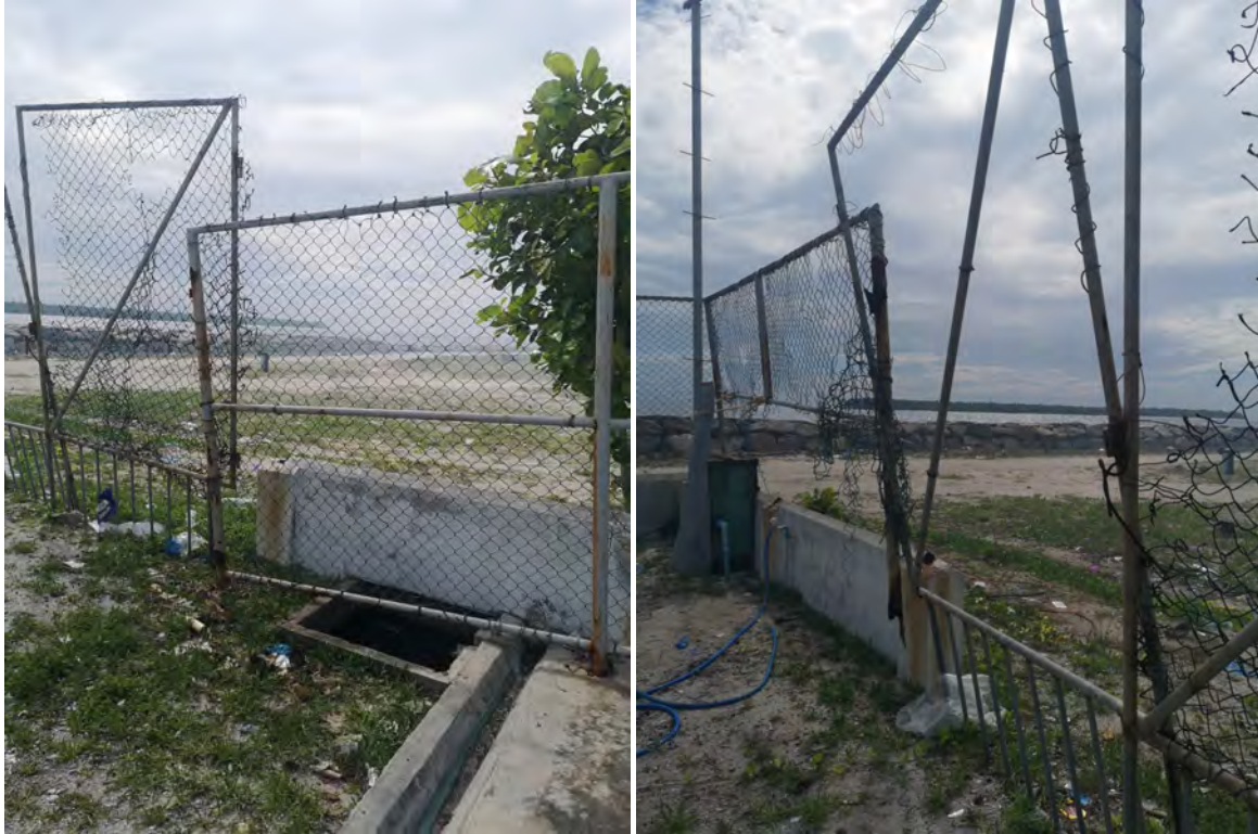
Figure 10 Broken down boundary fence of the IWMC site
