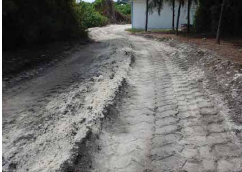
Figure 21: Impact on roads from heavy vehicle transport in an island in Maldives
