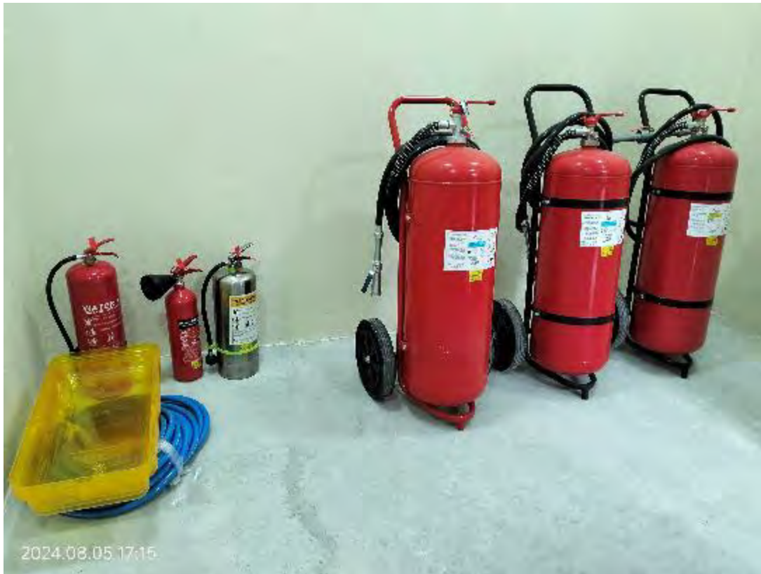
Figure 2. Photograph of fire extinguisher were installed on site.
