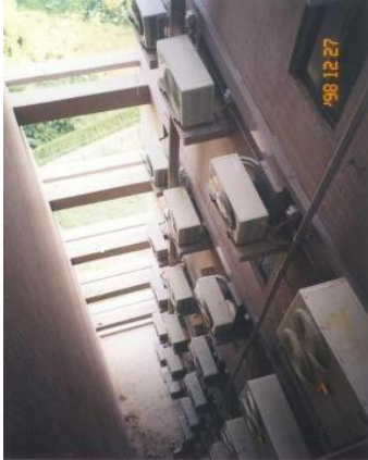
(a) Incorrect Placement
