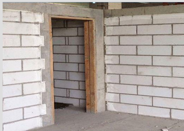
300 mm Autoclaved Aerated Concrete (AAC) with 15 mm plaster on both sides.U Value 0.54 W/m 2 K
