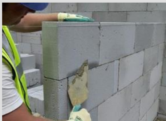
200 mm Autoclaved Aerated Concrete (AAC) with 15 mm plaster on both side .U Value 0.77 W/m 2 K
