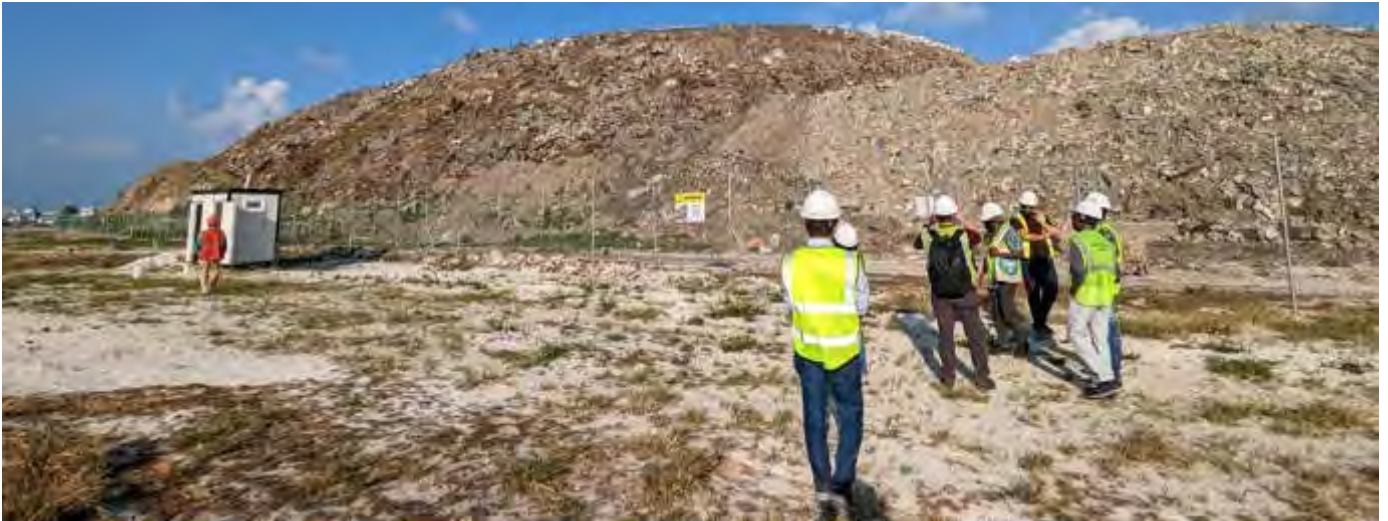
Photo 36 by Naif 27/02/23 16:57hrs Members of MOE, ER, D.B.O and E.P.C conducting a site walk around.
