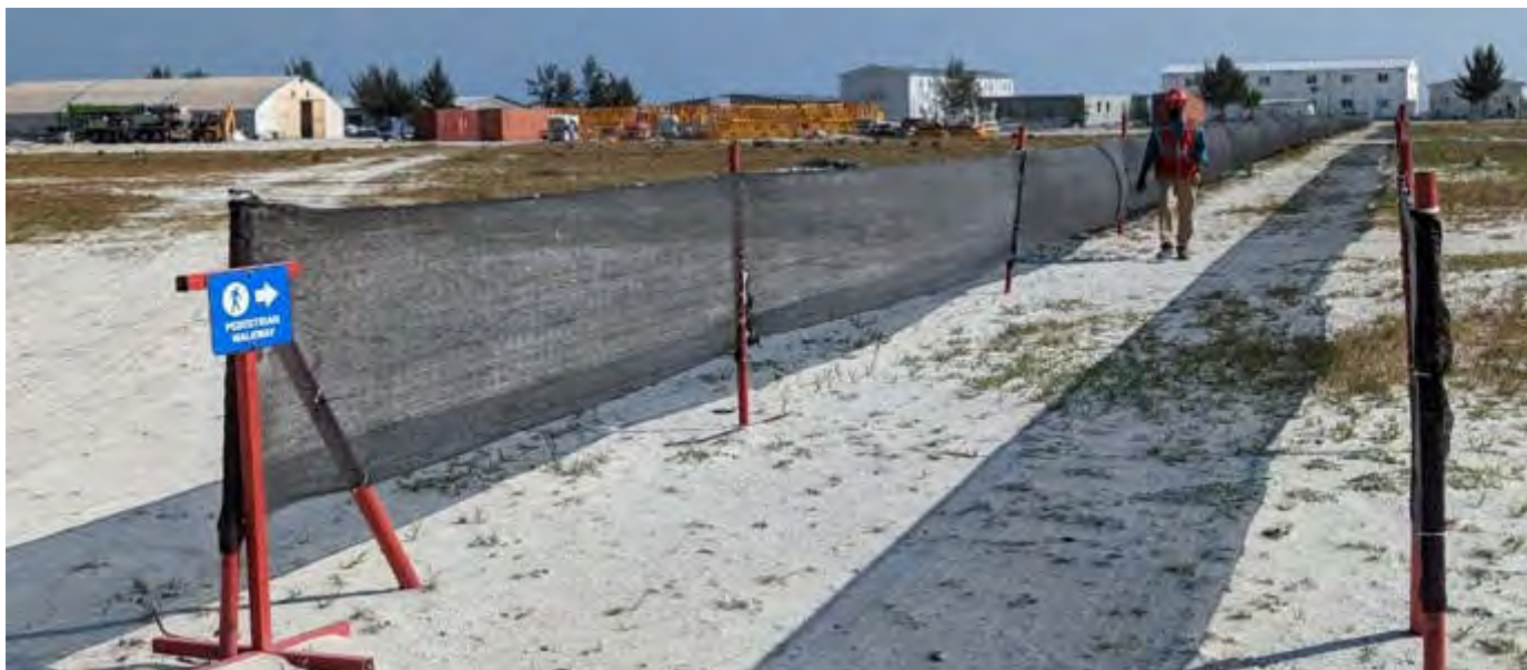
Photo 01 by Naif 27/02/23 15:33hrs. Pedestrian protected path from the site entrance to. Workers camp..
