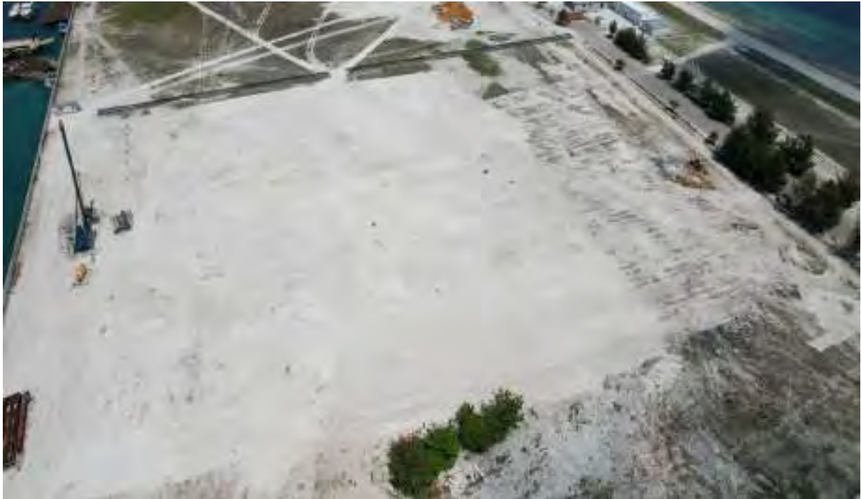
Stripping of the site by removing the vegetation of the site to be prepared for the piling activity is ongoing.
