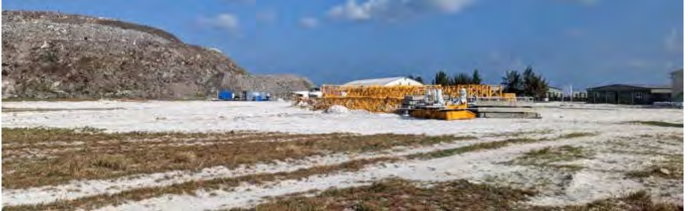
Photo 11 by Naif 27/02/23 16:02hrs. Tower crane delivered to site, yet to be setup and established.
