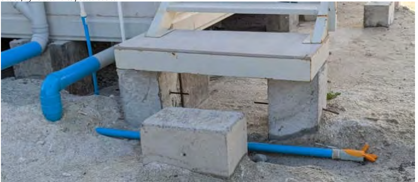
Photo 27 27/02/23 16:36hrs. Several tripping hazards, ground needs to be levelled off and pipes properly capped and secured.
