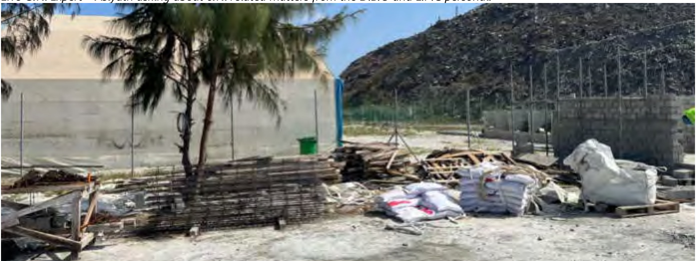
Photo 16 by Naahee 18/02/23 09:42hrs. Some construction materials on site for the temporary facilities construction work thats ongoing.
