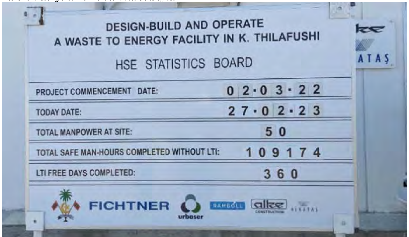
Photo 21 by Naif 27/02/23 16:26hrs. HSE statistics board established on site, outside the contractors site office.
