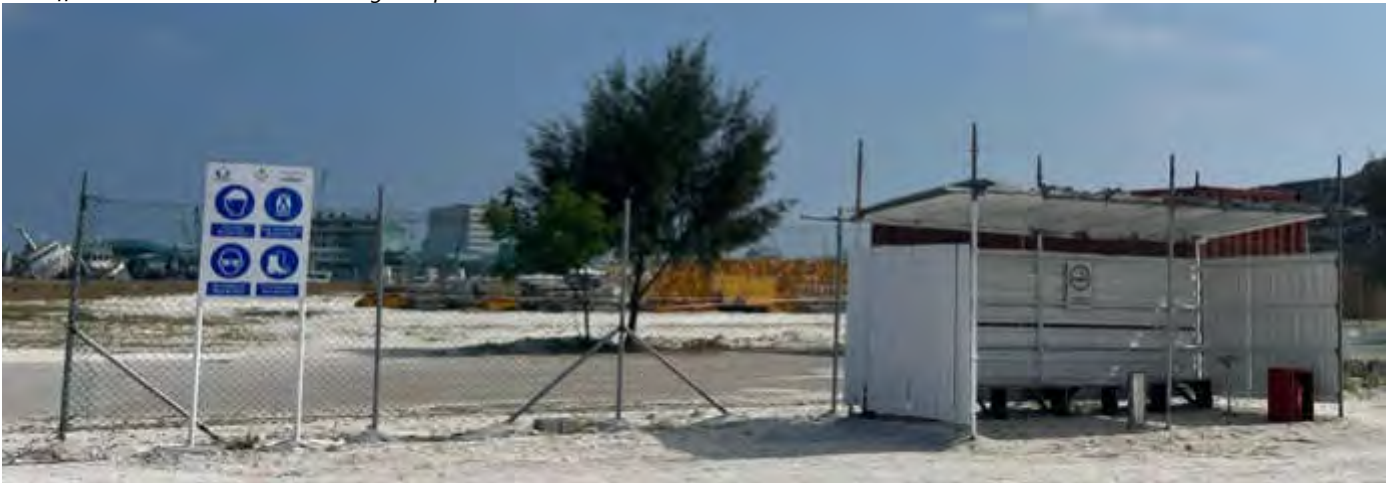
Photo 02 by Naahee 18/02/23 09:33hrs. Designated smoking area and safety signage around the site, workers area is separated by a fence within the site area.
