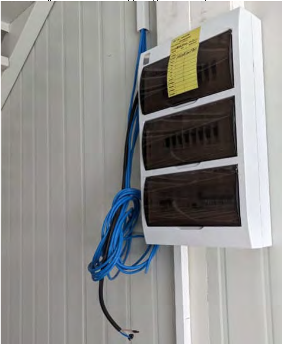
Photo 25 by Naif 27/02/23 16:35hrs. Electrical cables and communication cables not in use, should be secured properly.
