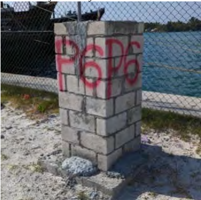
Photo 09 by Naif 27/02/23 15:58hrs. P6 survey control point established, several control points established around the site, these will remain in place until completion of project.
