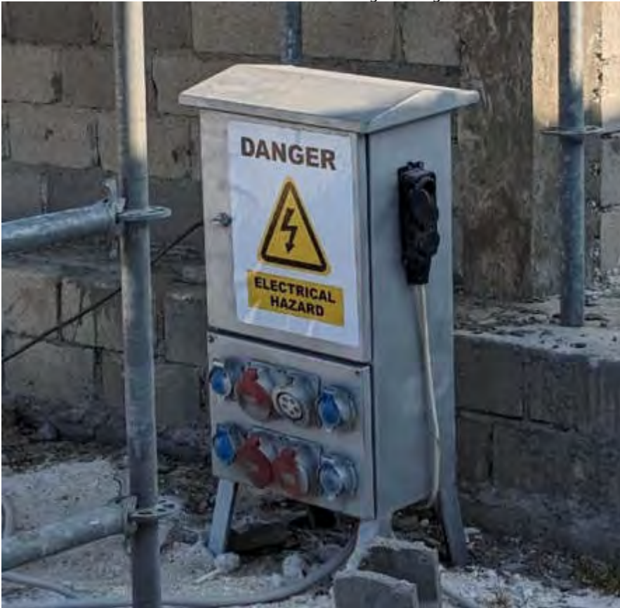
Photo 31 by Naif 27/02/23 16:42hrs Temporary electric distribution board in use, the stands require to be higher for safety, from flooding, and checked regularly for water proofing. Some sockets seen here are not waterproof.
