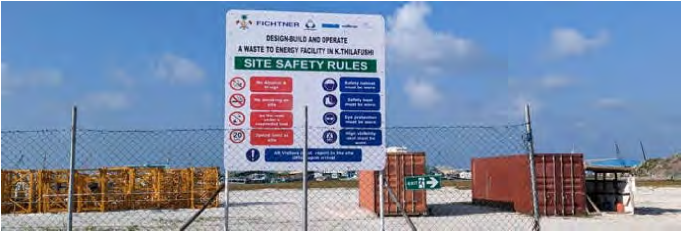
Photo 26 by Naif 27/02/23 16:36hrs. Site safety related rules posted at site.
