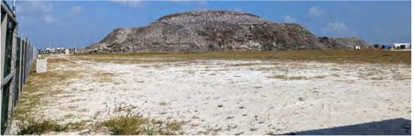
Photo 04 by Naif 27/02/23 15:40hrs. WAMCO landfill and fencing works incomplete.
