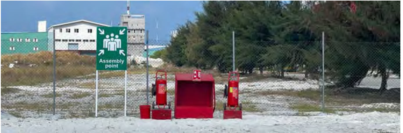
Photo 06 by Naahee 18/02/23 09:36hrs. Assembly point setup and fire fighting equipment placed.
