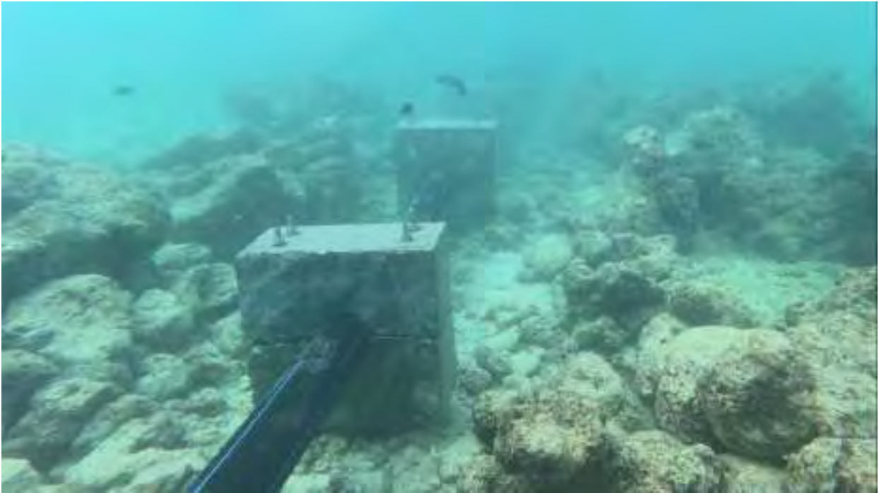
Outfall Pipeline installation to discharging sewage from WWTP to the sea was completed.
