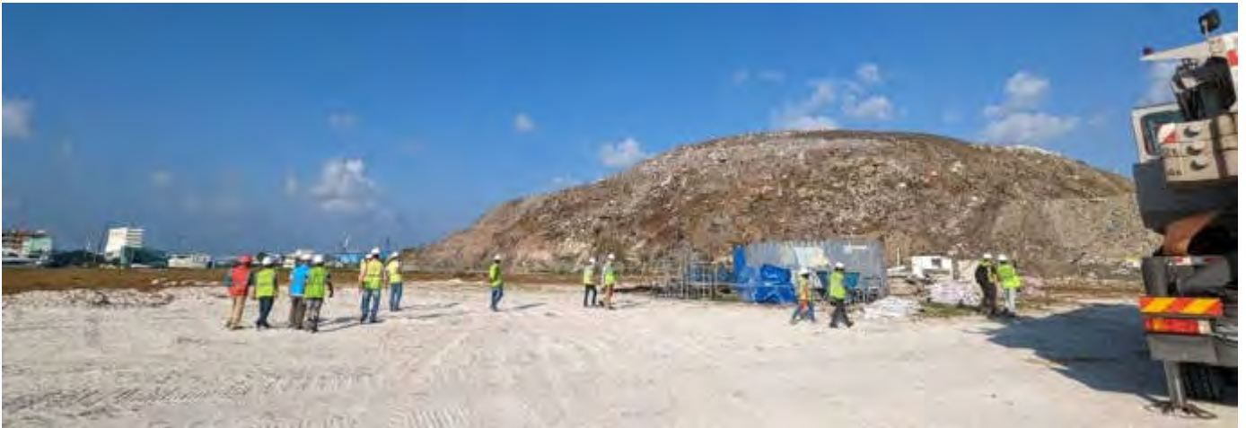
Photo 37 by Naif 27/02/23 17:00hrs Members of MOE, ER, D.B.O and E.P.C conducting a site walk around.
