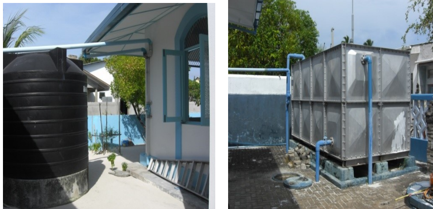
Water storage tanks used in Maldives
