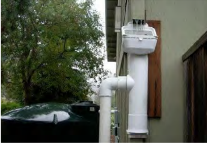
Rain head and First flush diverter
