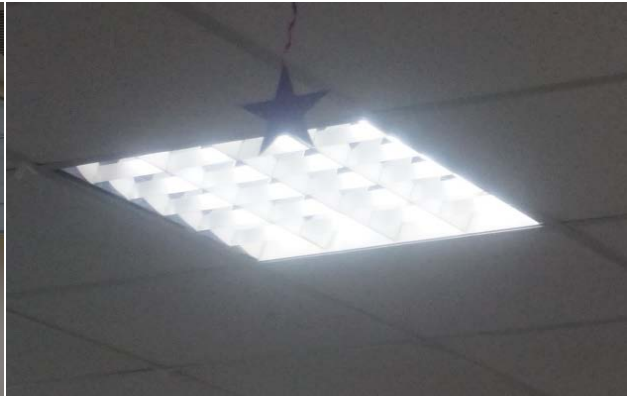
Figure 1-36: T8 Tube Diffuser in Velaanaage – 144W LED
