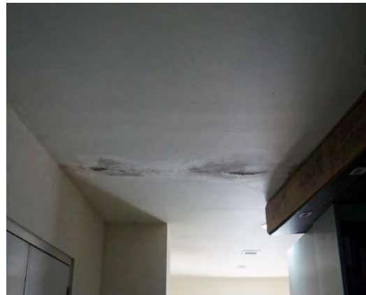
Figure 1-34: Image above shows damaged ceiling from air conditioning system water leakage
