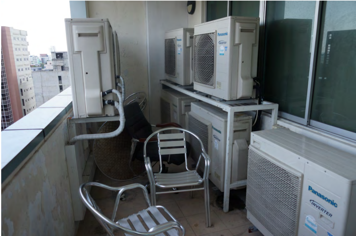
Figure 1-28: Outdoor air conditioning units at Velaanaage building
