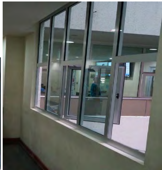
Figure 1-32: Image above showing windows open during office hours at Velaanaage Building
