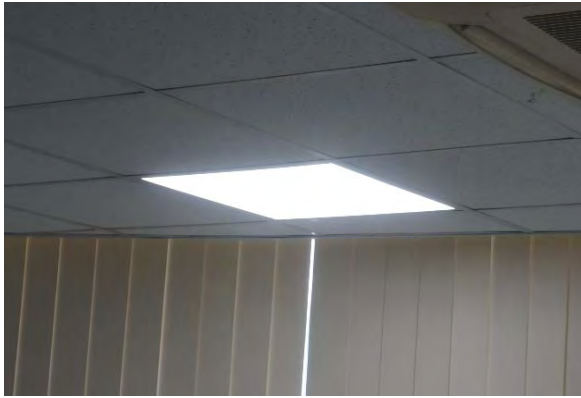
Figure 1-35: LED light panel– estimated 33W
