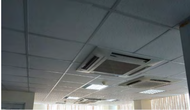
Figure 1-31: Image above internal air conditioning units in a duplicate arrangement
