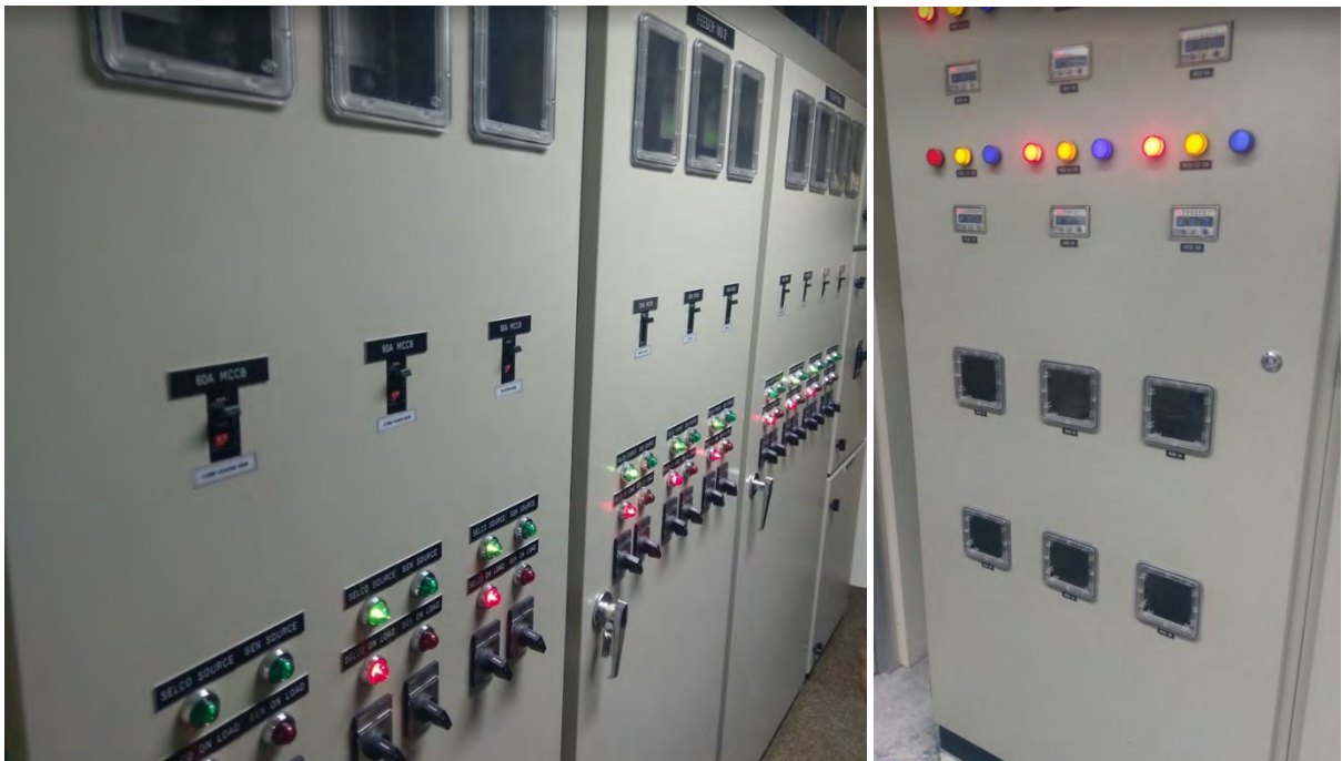
Figure 1-44: Existing main power distribution board at Velaanaage office building
