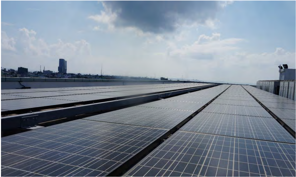
Figure 1-43: Existing PV array on Velaanaage office building
