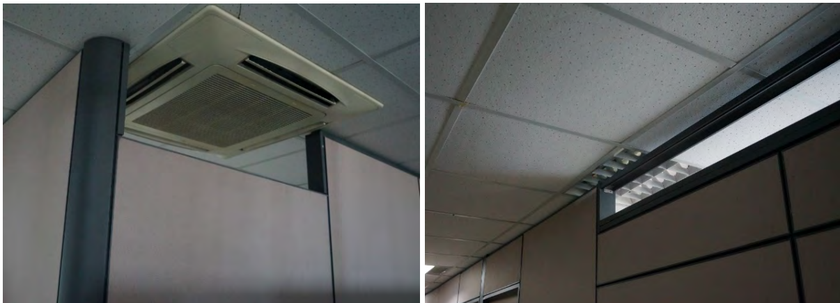
Figure 1-33: Images showing internal air conditioning units
