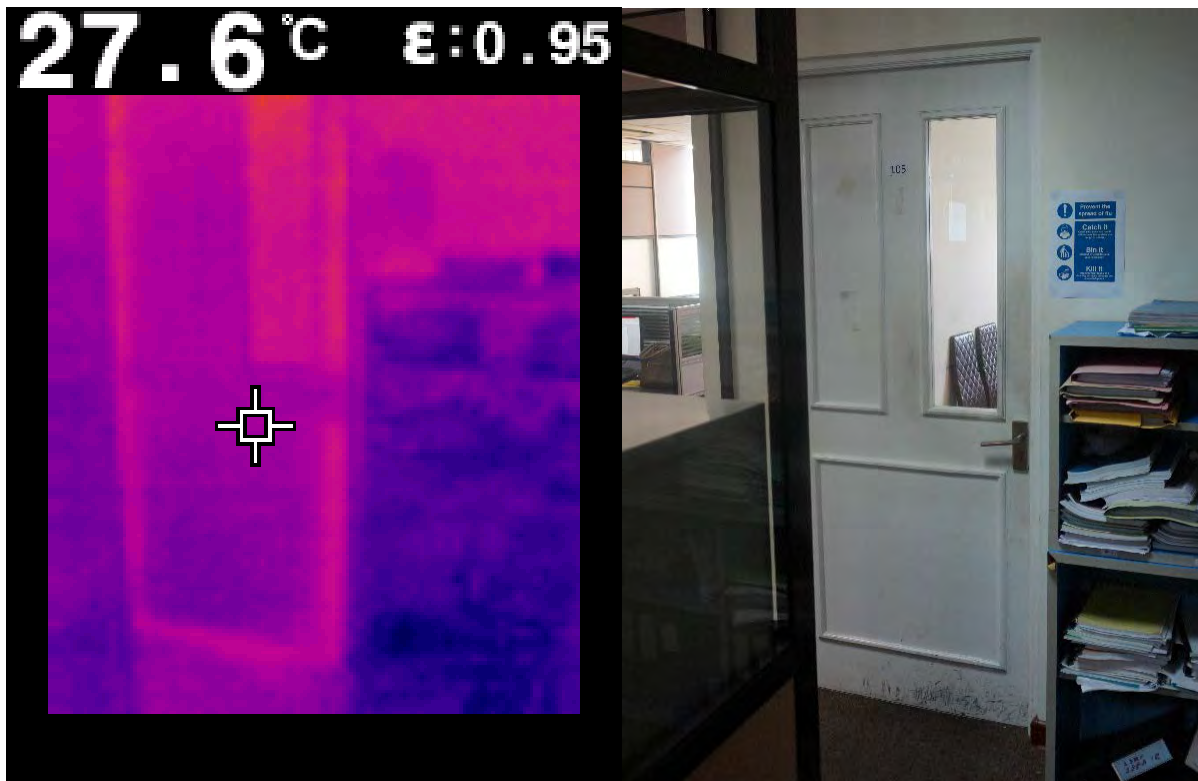
Figure 1-27: Typical team preparation room with thermal image for the same room
