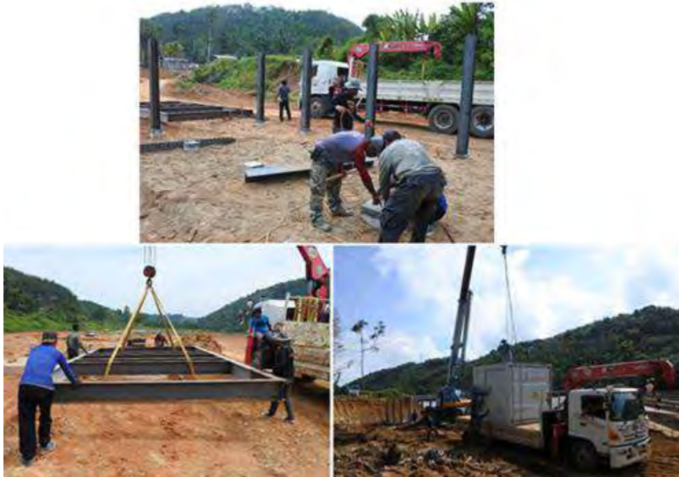
Figure 3-14: Installation of transformers (reference pictures of similar works)
