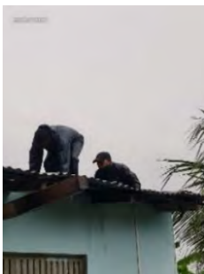
Figure 48: A roof of the house in S.Hithadhoo was blown away. Image courtesy: MNDF
