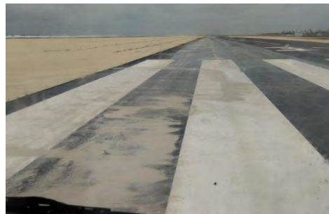
Figure 47: Ha.Hoarafushi Airport runway. Some part of runway is filled with dust due to strong winds on 25th July 2021. Source: http://mihaaru.com/business/94900
