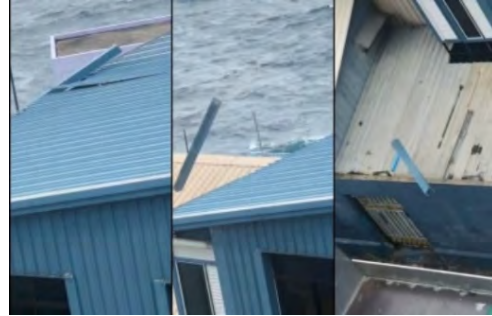
Figure 45: An image showing the Maldives ports limited building roof, which was blown away due to strong on 25th July 2021. Source: https://dhen.mv/105511
