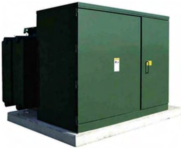
FIGURE 8 TRANSFORMER ON CONCRETE SLAB
