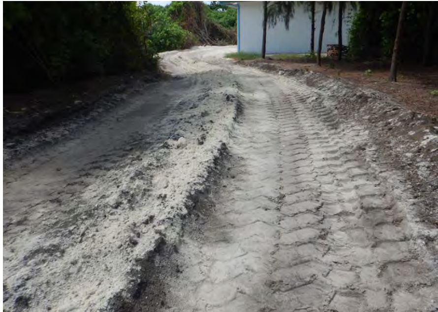
Figure 19 Impact on roads from heavy vehicle transport in an island in Maldives
