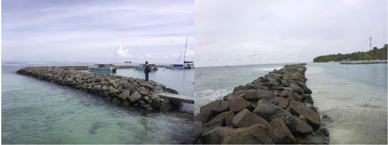
Figure 4.10 Current break water design for harbours – Raised rock boulder breakwater in Rasdhoo and Maalhos
