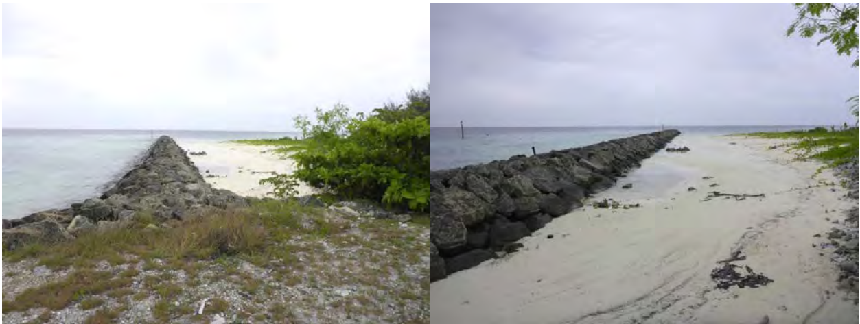
Figure 4.13 Groyne constructed in Feridhoo to prevent sedimentation in harbor basin and to prevent erosion
