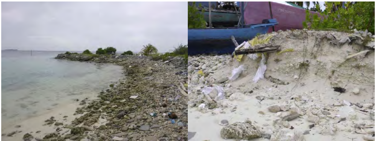
Figure 5.4 Erosion on the western side of the harbor
