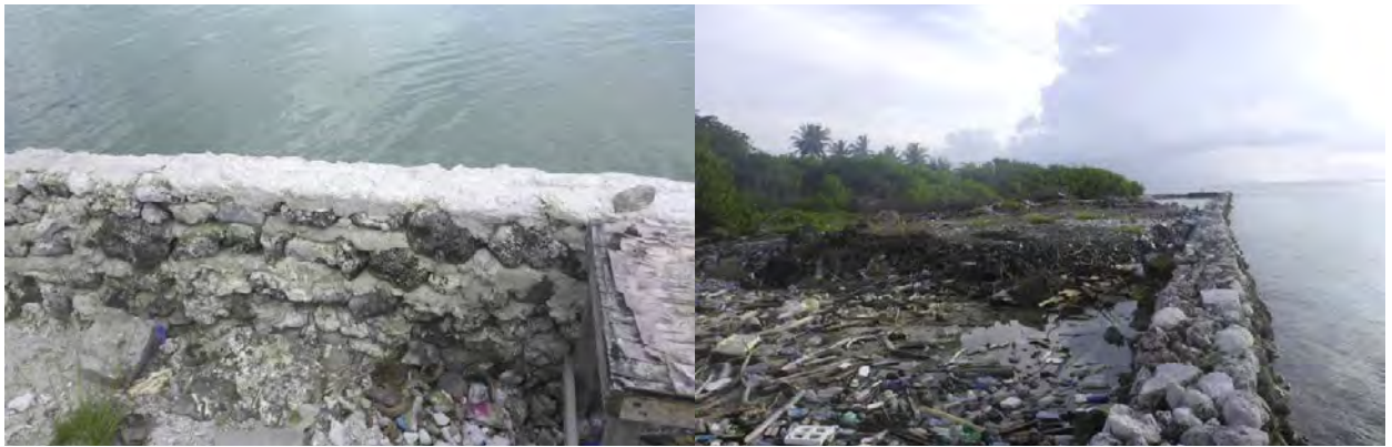
Figure 4.5 Examples of Seawall structures: semi-plastered coral mound seawall in Bodufolhudhoo and Mathiveri
